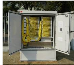
Fiber distribution terminal (FDT)
