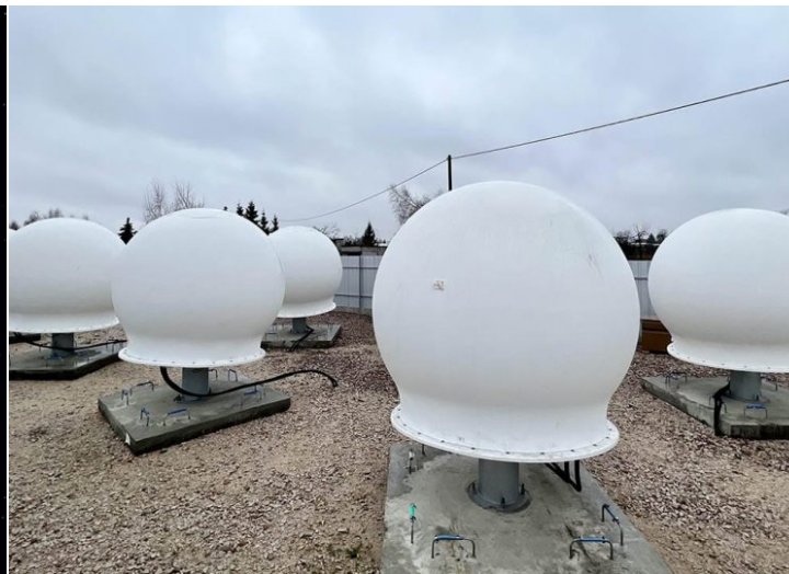
Starlink Ground Station Antennas
